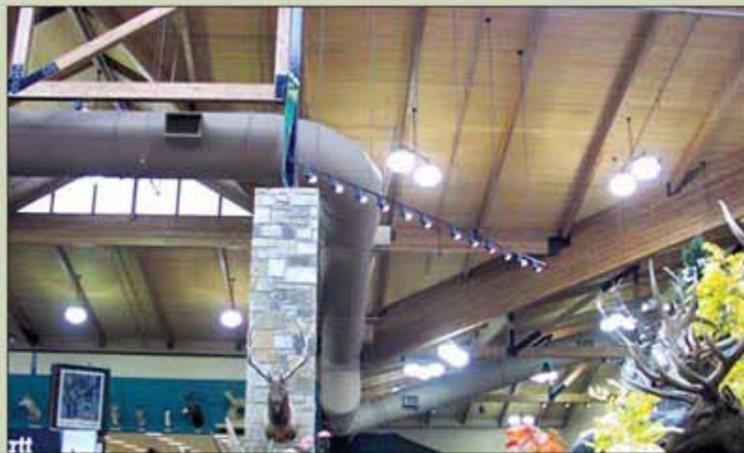
The finished, visible spiral ductwork from ground level.
