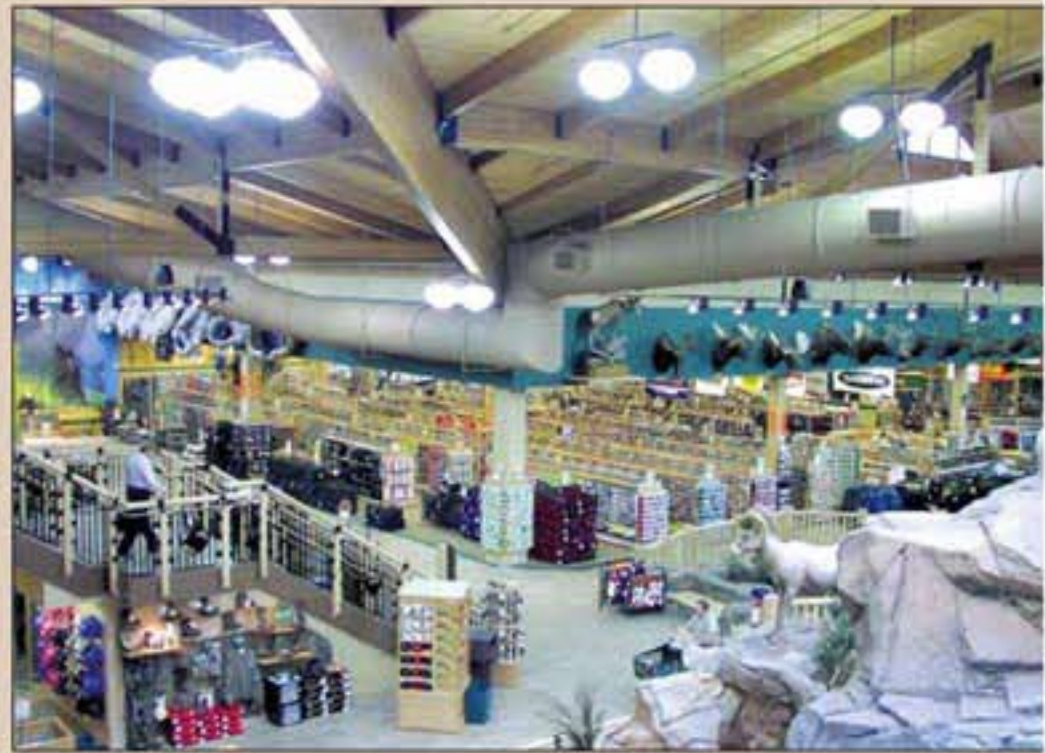
The ductwork hangs far above the store below.
