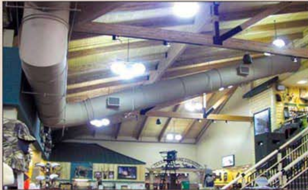
The spiral ductwork mounted in the Fort Worth, Texas, store. The taps were shop-mounted parallel to the floor at a 17 1/2- and 5 1/2-degree roof pitches.
